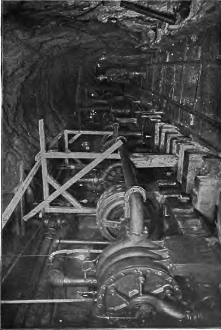
PLATE 93.—View of Three Six-stage Worthington Centrifugal Pumps—Motor Driven—Used in Tunnel Near Shaft 4. This pump had capacities of 700, 600, and 540 gallons per minute under 500 foot head. They pumped continuously for nearly two years from 2200 to 1100 gallons per minute.
